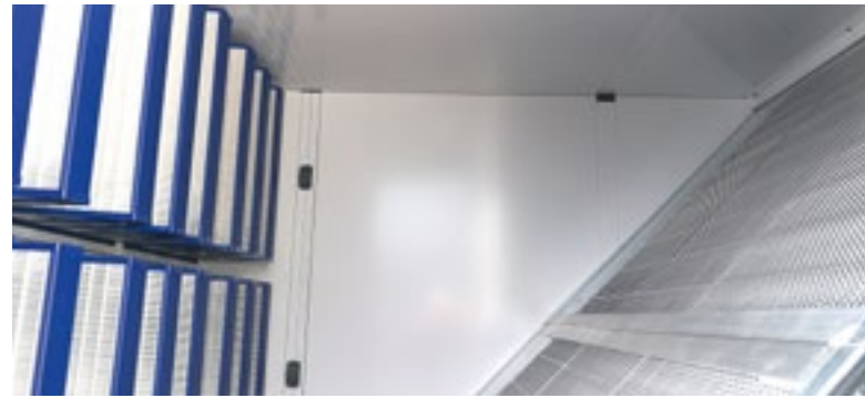
54 TROX H13 HEPA filters are used.
