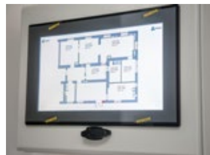
A defined and monitored overpressure hierarchy is mandatory in the laboratory building.
