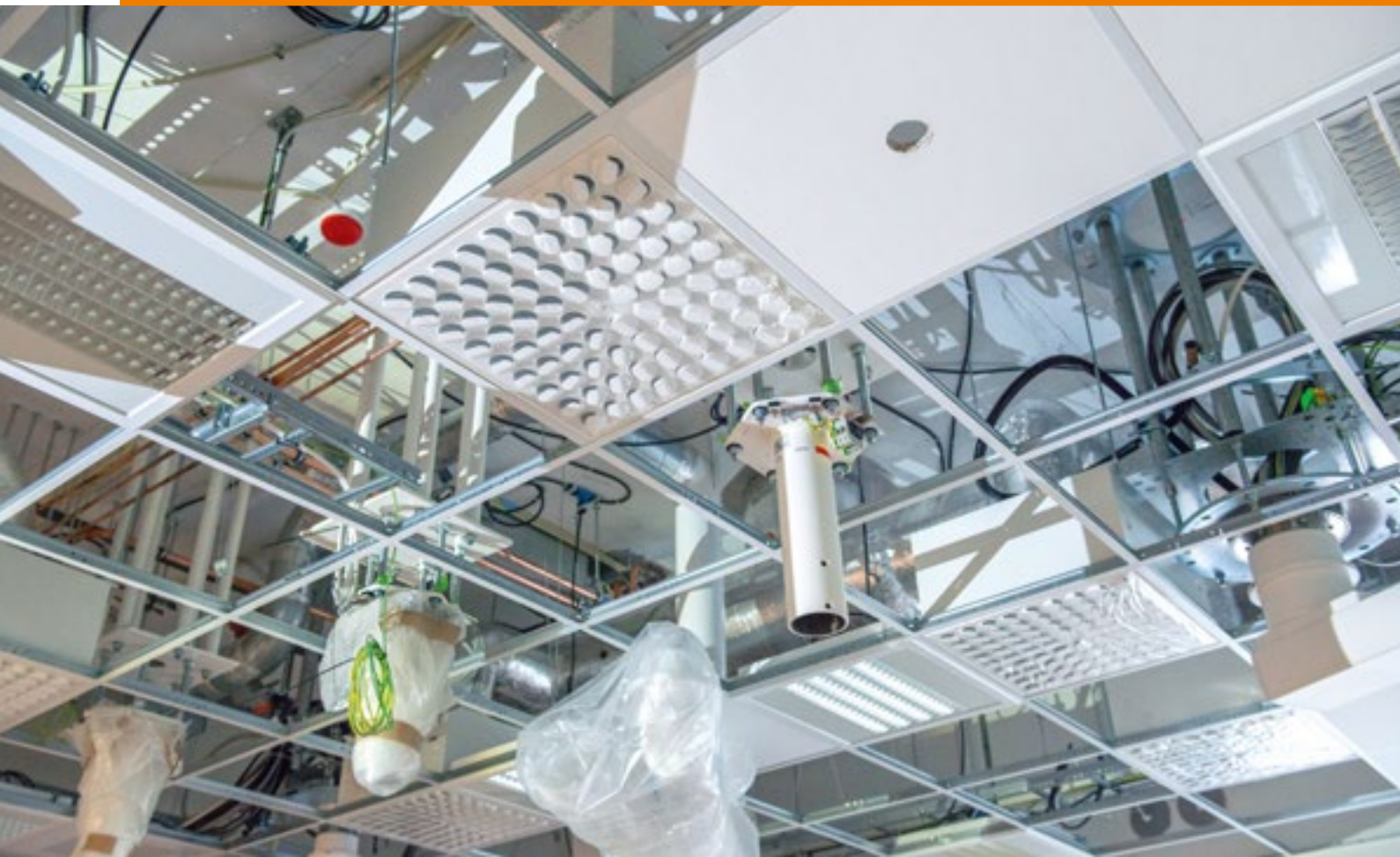
TFC ceiling mounted particulate filter with Opus front design in the operating theatres and corridors.
